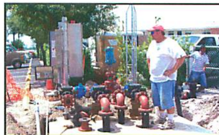
(RIGHT) Tony Bowers, Project Manager for RK, looks over the progress. (FAR RIGHT) The new station is set up on a by-pass until cut over is completed.
