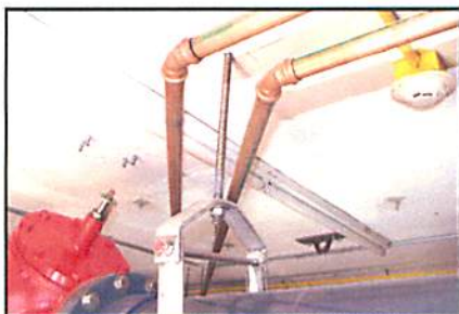
(ABOVE) Viega copper press fittings were used on all tube under 2".
